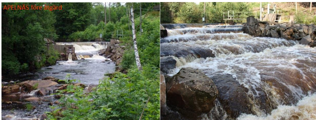
Bypass through the dam in the Atlantic salmon river Rolfsån. Before (left) and after (right). The former technical fishway did not function properly. Photo by Andreas Bäckstrand
