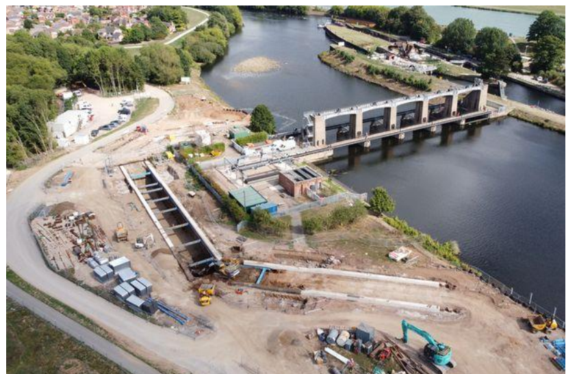
£8.5m Holme Sluices deep vertical slot fish pass under construction on the River Trent a recovering salmon river
