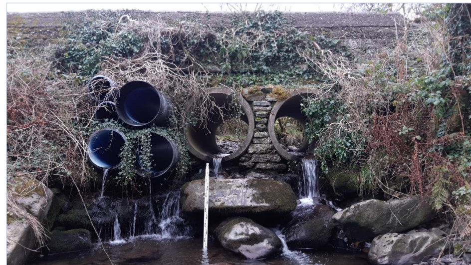
Culvert impeding fish migration (Credit: B. Coghlan (IFI))
